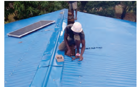
Picture 6. A new roof and new ceiling tiles were installed at Mercy Home in 2021.
